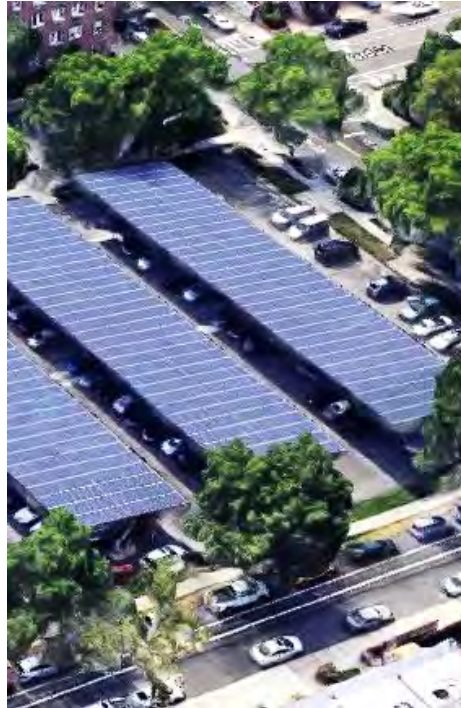
Solar awnings over parking lots
